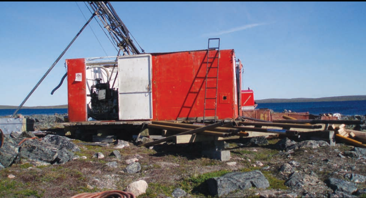
Geotechnical drilling in area of proposed Goose pit, Meadowbank Project. PHOTO BY K. COSTELLO
